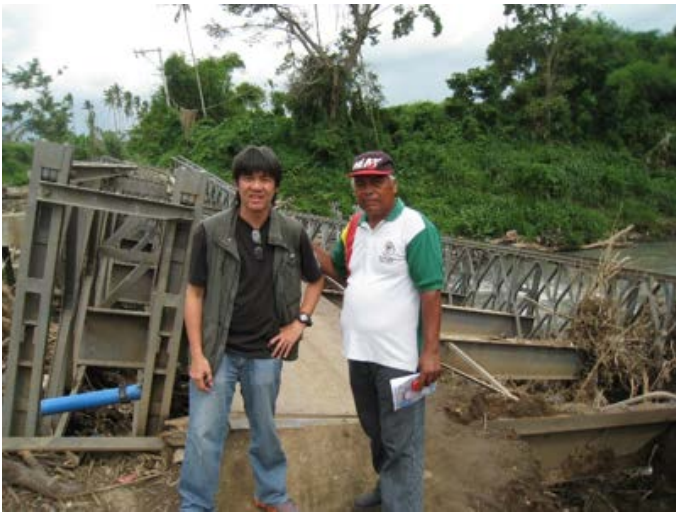
Stefan at broken bridge at Bukal after Typhoon Glenda
